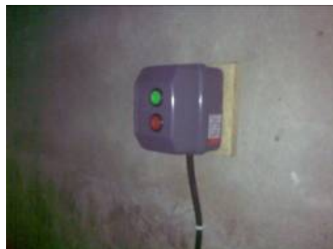
Motor starters installed for the 3 machines
