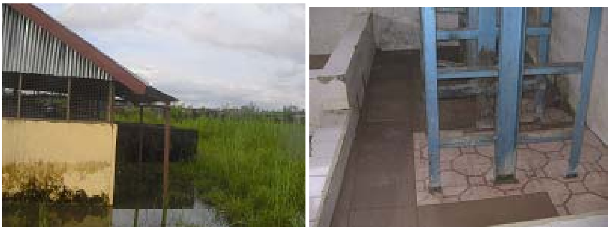
Figure 1: Roof projected, and presser base and cassava mash packing trough tiled at Bomadi
