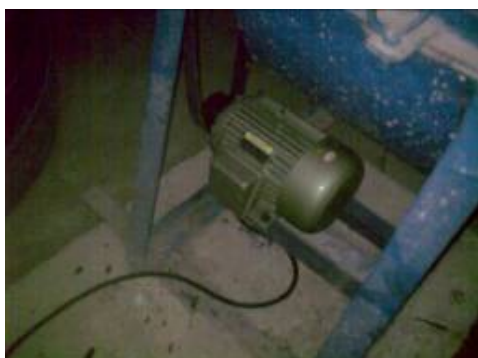
Figure 9: 5 hp, 3 phase electric motor drive
